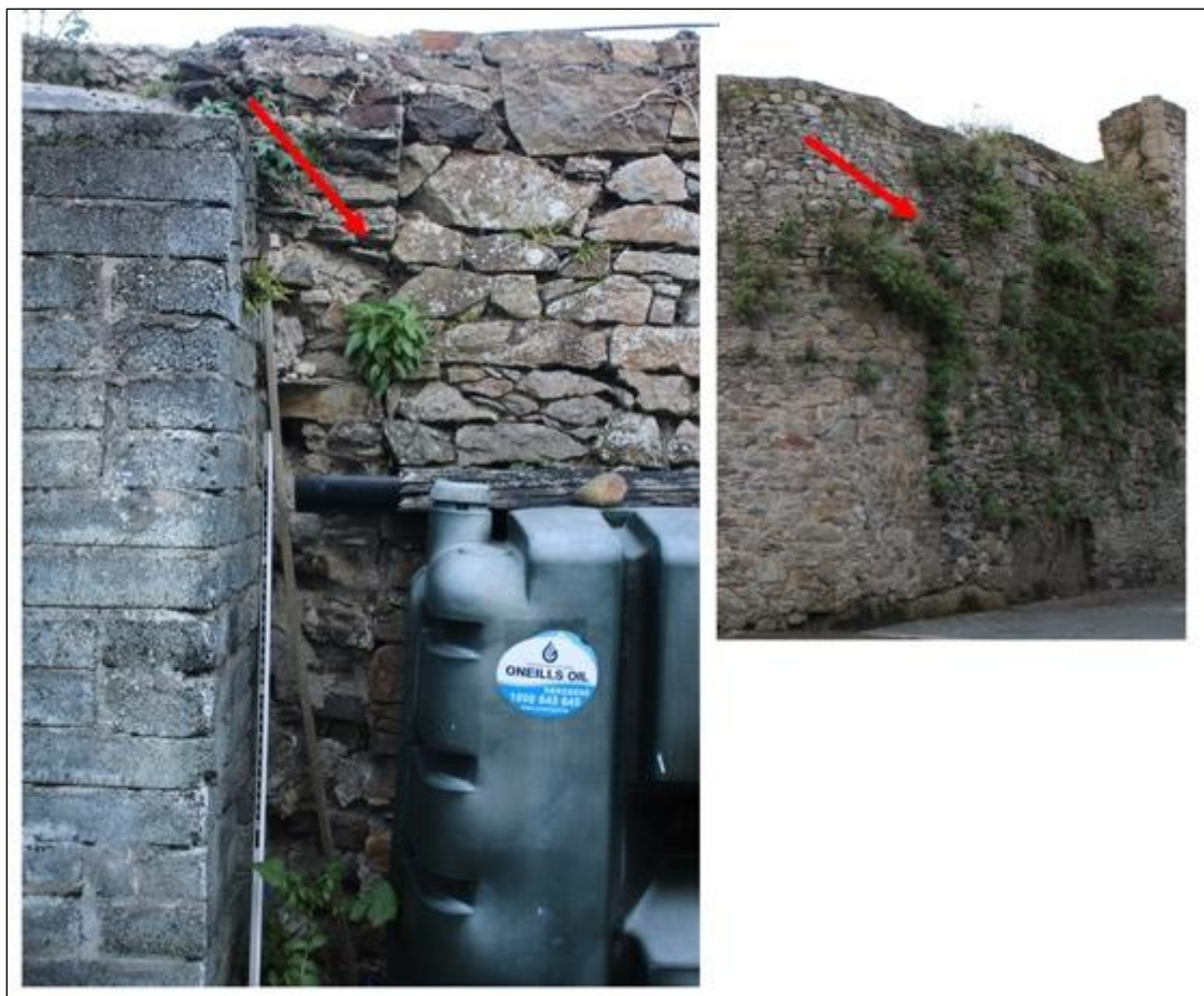
Plate 25: Left photo, west facing section of wall which appears to run west and note the abutting curtain wall to right. Right photo, northeast facing section of wall note bulge in masonry at this point.
