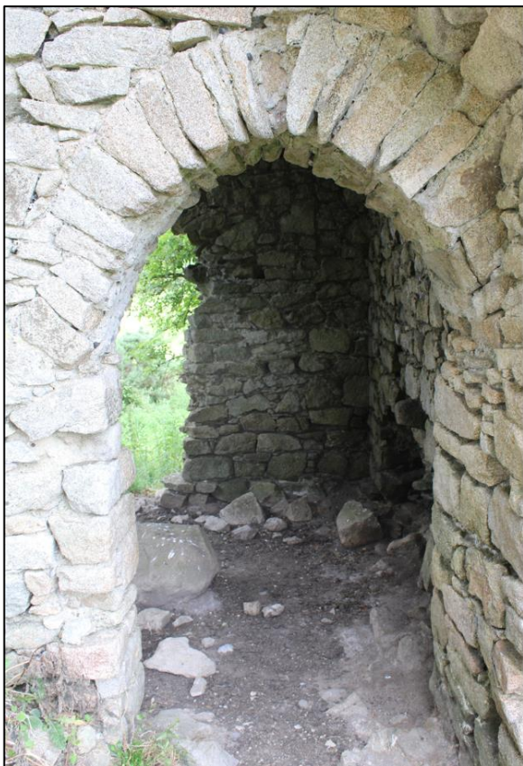
Plate 58: Clonmore Castle note mortar and stone floor surface.
