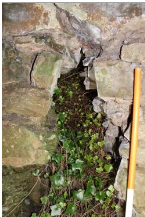
Plate 35: Collapsed section on masonry in north section of wall in tower.
