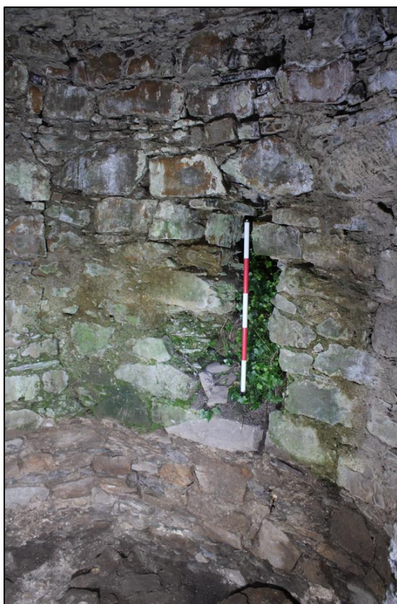
Plate 55: Crack in tower at garderobe.
