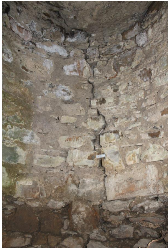
Plate 60: View of second crack in NW face of tower.
