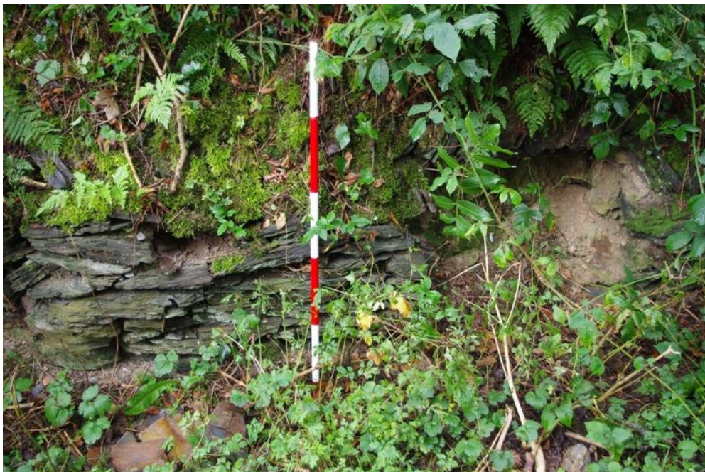
Plate 18: Detail showing extracted bedrock used to construct a drystone wall at the side of the rock-cut ditch west of the castle. It is likely that this feature is contemporary with the construction of the castle (photo: Ivor Kenny).
