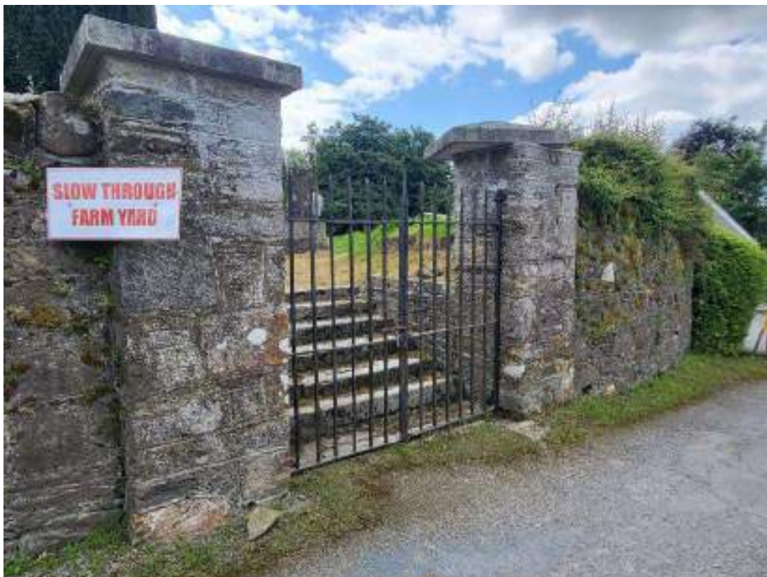
14. North Graveyard wall entrance (Note dislodged pier cap)
