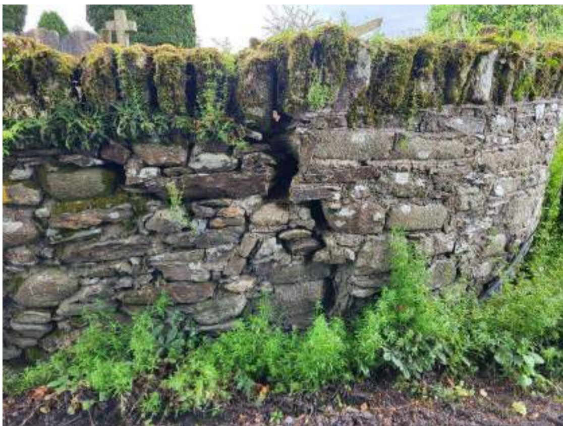
17. Serious crack in the wall at the south-west corner.
