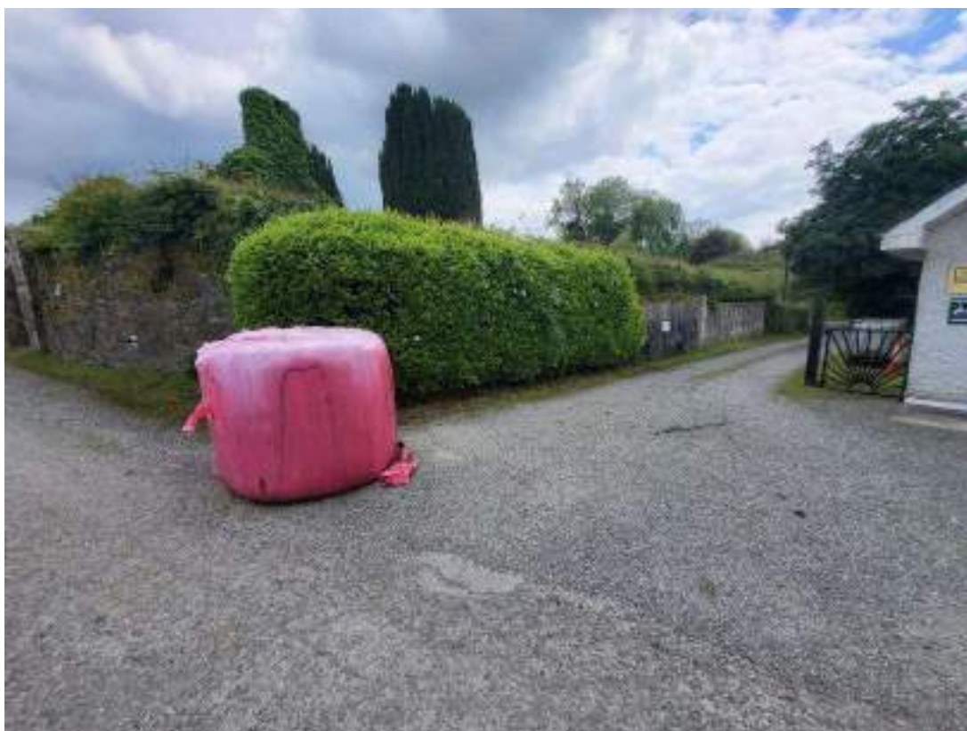
15. West graveyard wall, north end (Note vegetation)
