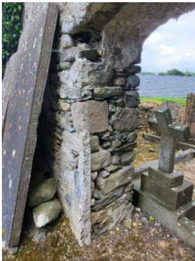
3. Door Reveal in West Wall (Note mortar wash out)
