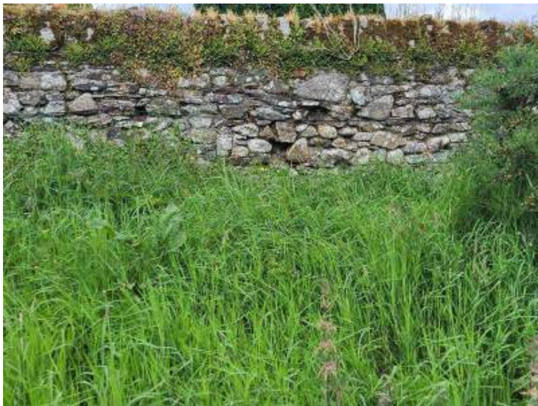
20. South Graveyard wall. (Note local damage)
