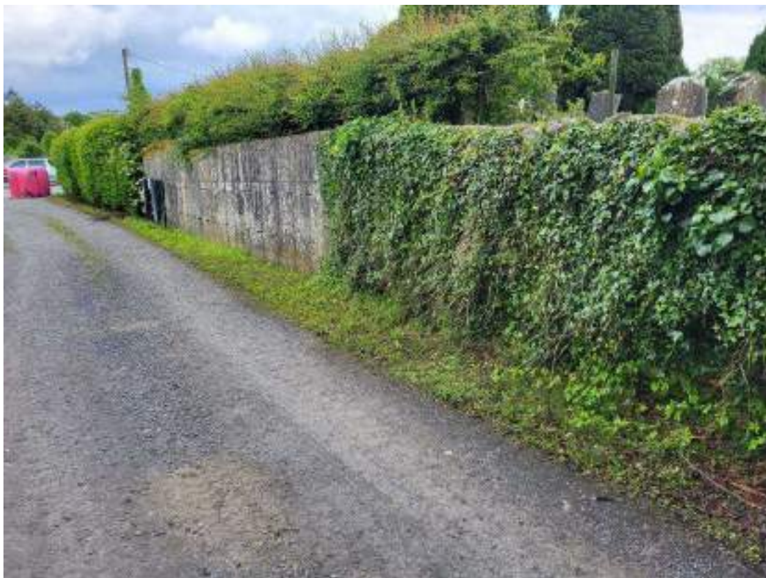
16. West Graveyard wall, south end (Note concrete replacement in central section).
