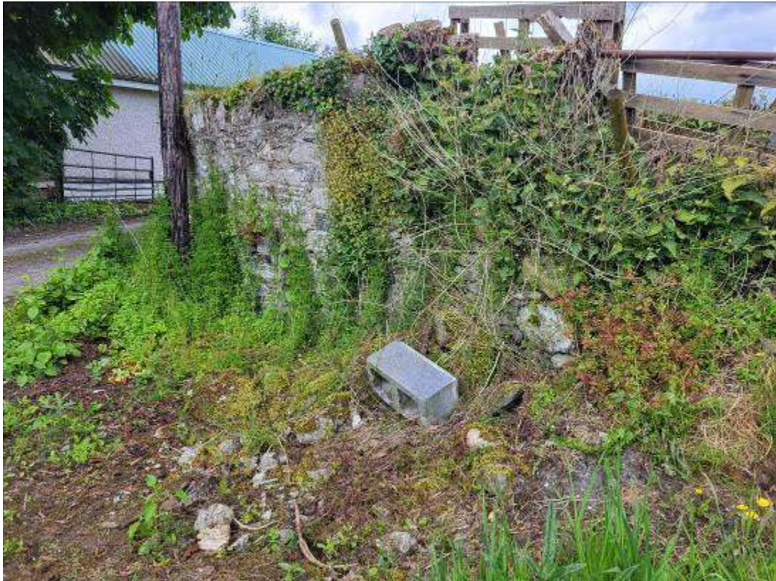
22. Leaning perimeter wall at Southwest corner of the graveyard
