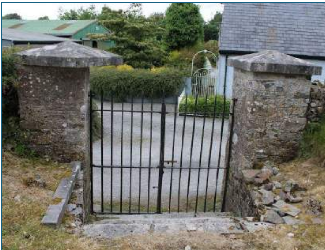
Plate 11: Entrance to the graveyard note pillar on gate is dislodged.
