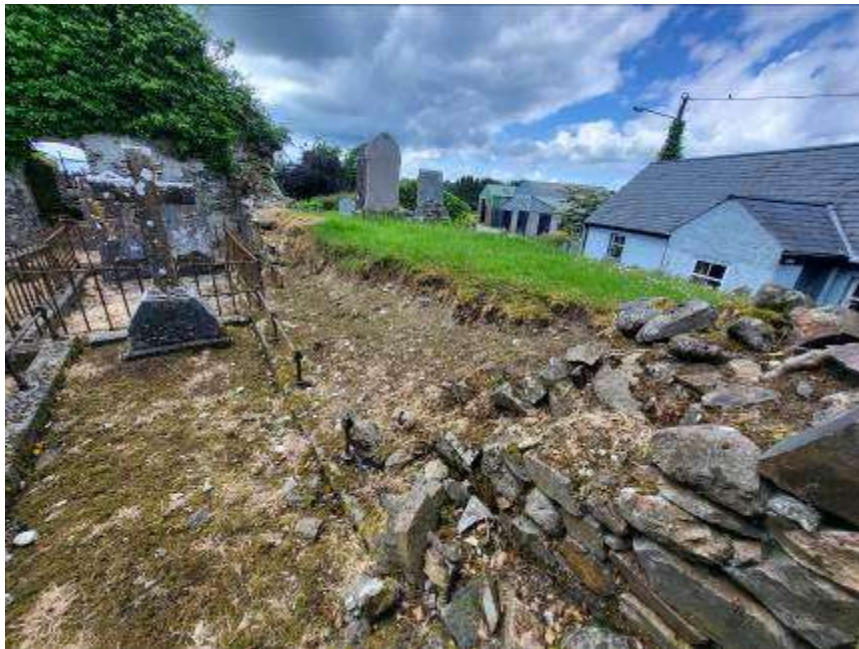
19. Destroyed North wall (remnants survive at both ends)
