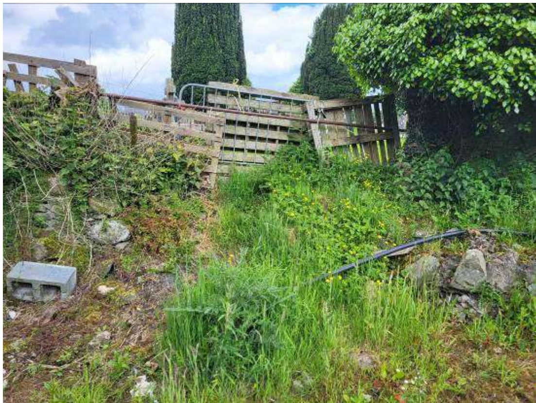
23. Section of collapsed South graveyard wall
