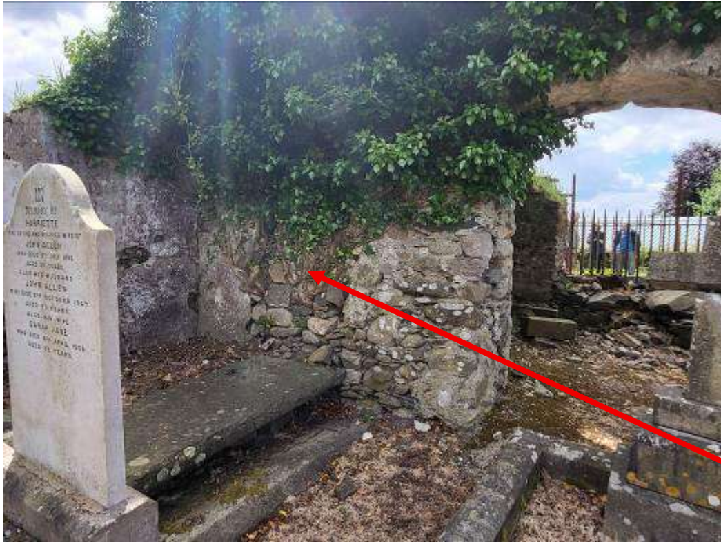
7. Detail of West wall interior (before removal of vegetation). Note area of damaged masonry
