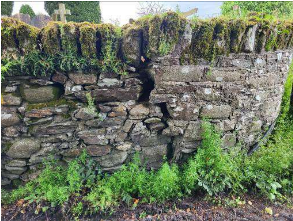
21. Fracture at leaning perimeter wall at the Southwest corner of the graveyard
