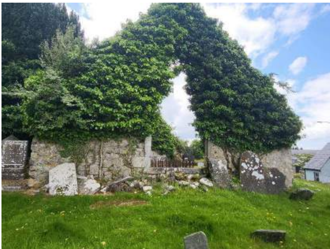
9. East Wall (Note heavy vegetation and fallen rubble)
