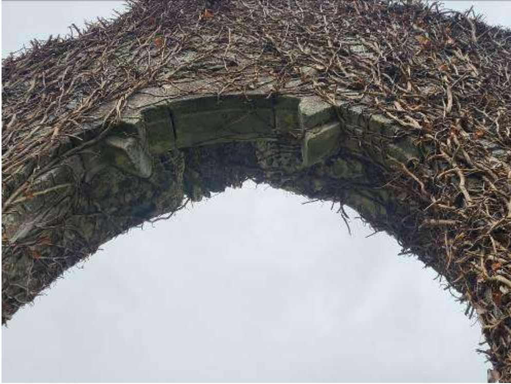
11. Tracery remnant on East window soffit
