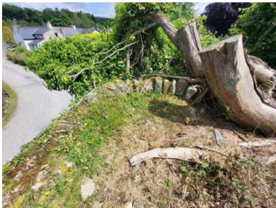
21. North-east corner of the Graveyard. (Note ground level is at the top of the wall)
