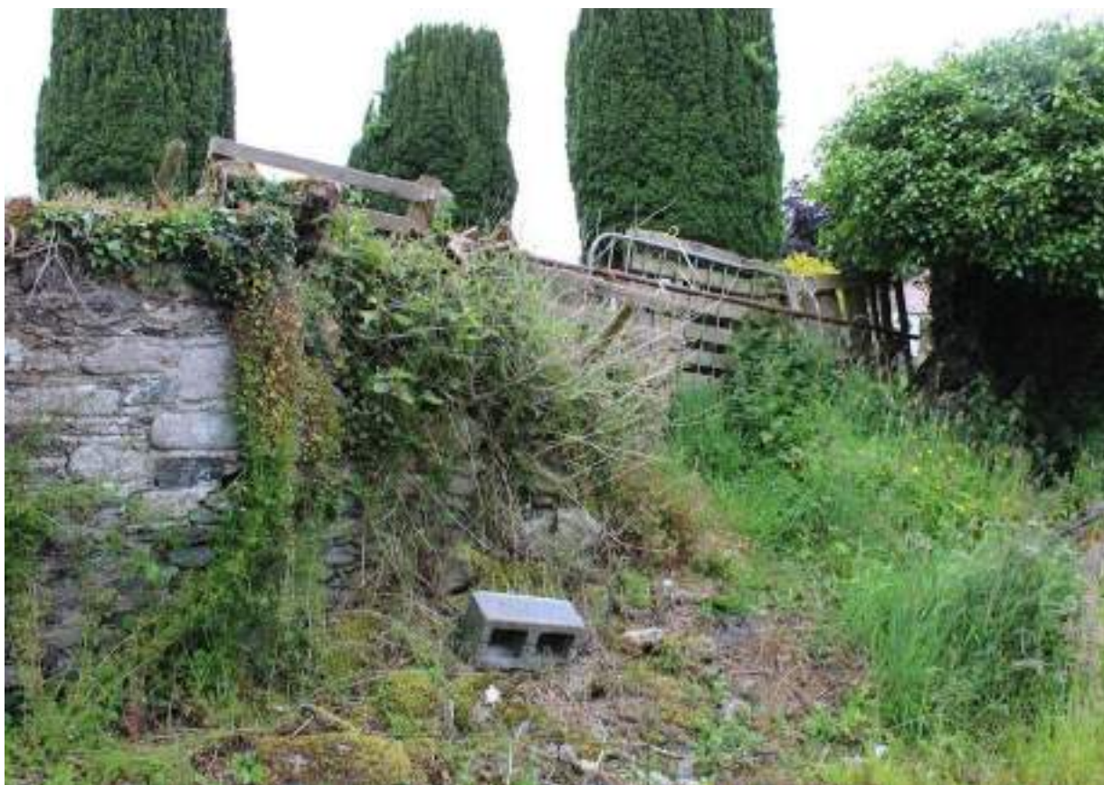
Plate 45: Southwest corner of the graveyard wall which has collapsed.
