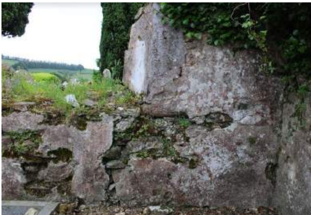
Plate 28: South wall of the church with evidence of window and plaster.
