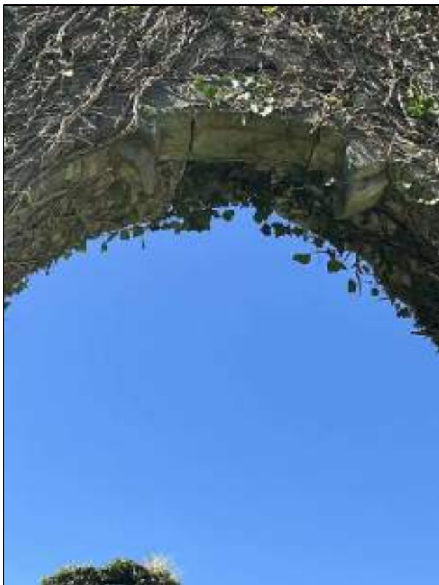
Plate 60: East window of church with intact granite voussoirs and possible remnants of tracery.
