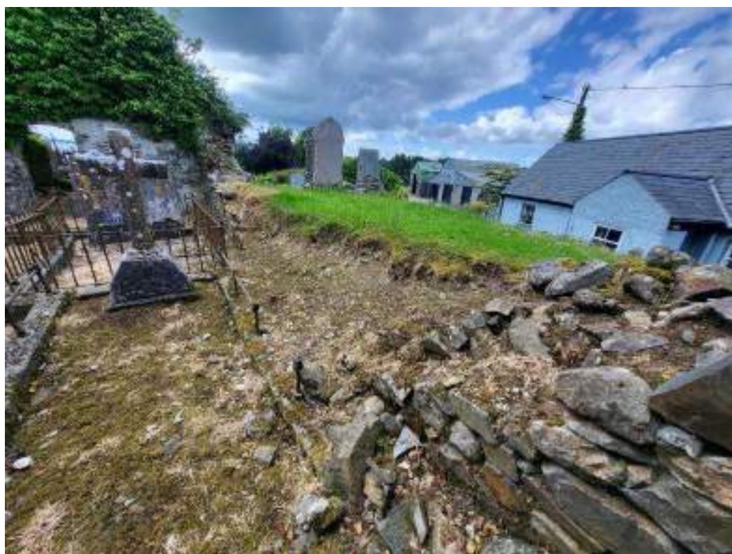
12. View of ruined North wall.
