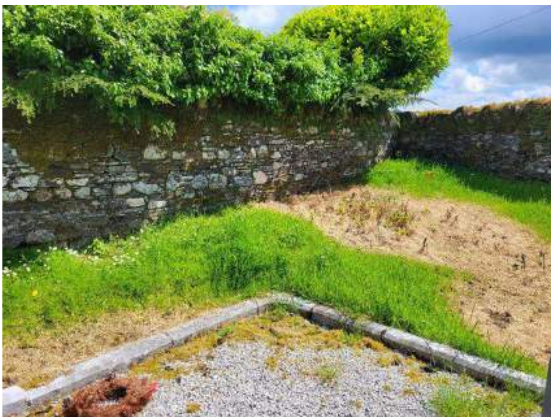
23. East Graveyard wall (Note severe leaning)
