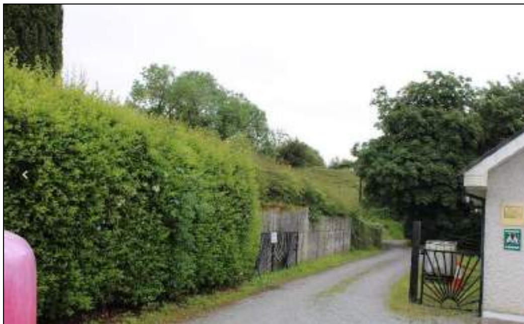
Plate 47: Concrete retaining wall on west boundary of the graveyard where the houses which were visible at the time of the first and third edition map were located/
