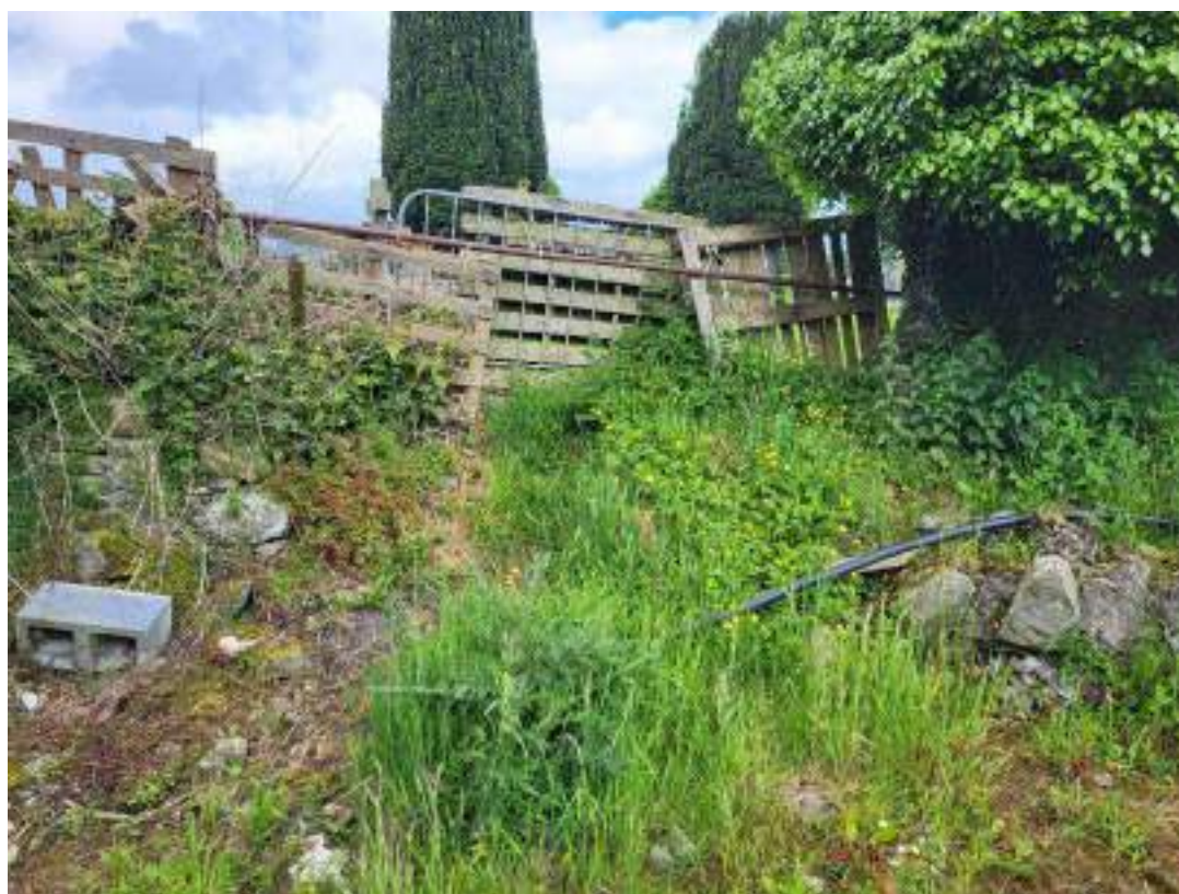
19. South Graveyard wall collapsed at the west end.
