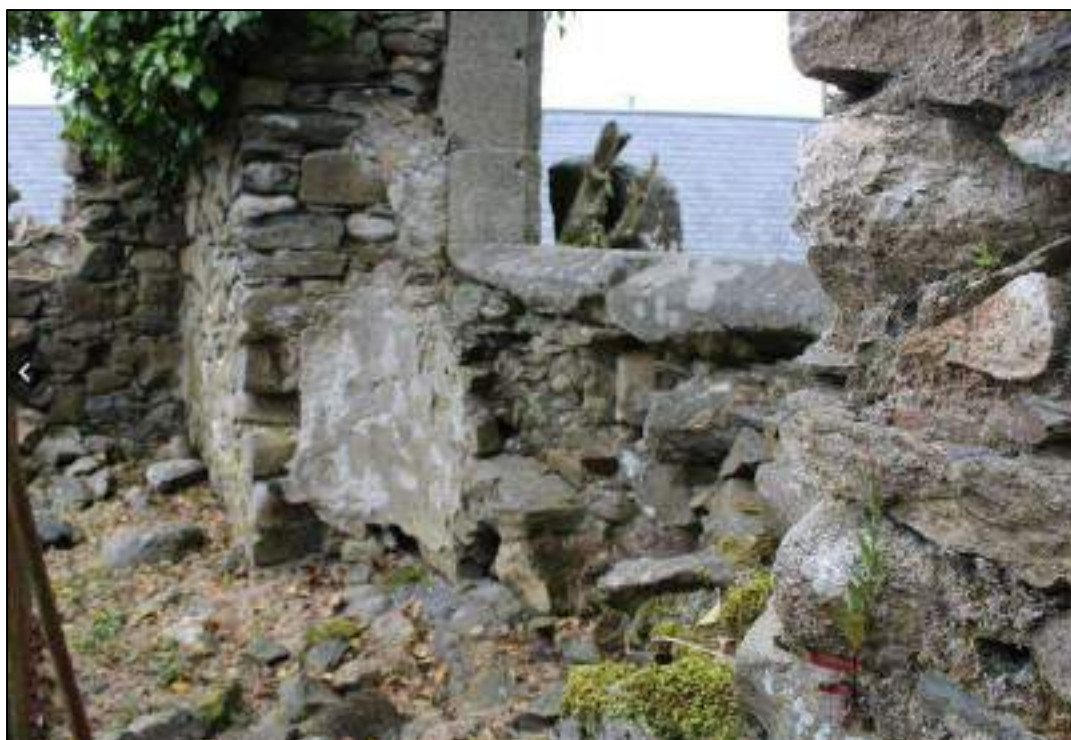
Plate 36: View of collapsed masonry at base of window in east gable.
