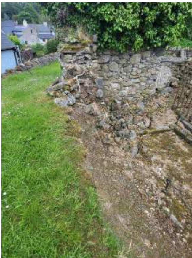
11. East Wall, north end and North wall east end (Note collapsed masonry under windowsill, and earthen bank on the line of the North wall).
