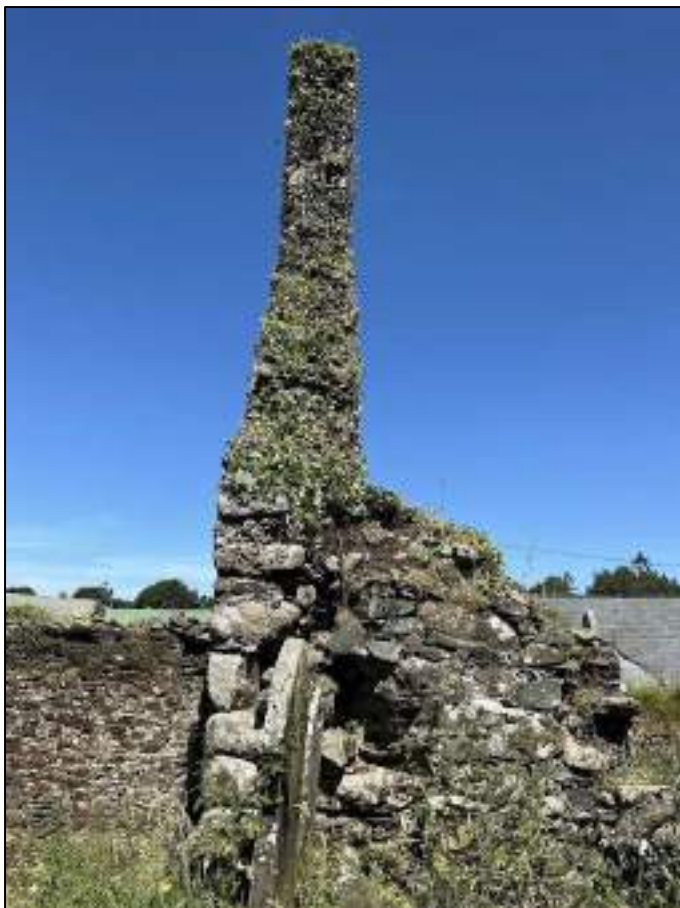
Plate 54: South wall of church and west gable, note the missing masonry.
