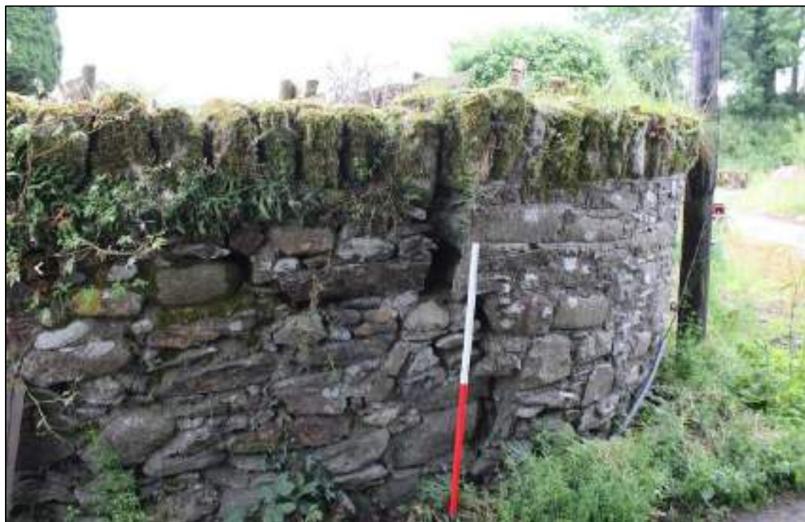
Plate 46: Crack at southwest corner of the graveyard boundary wall.
