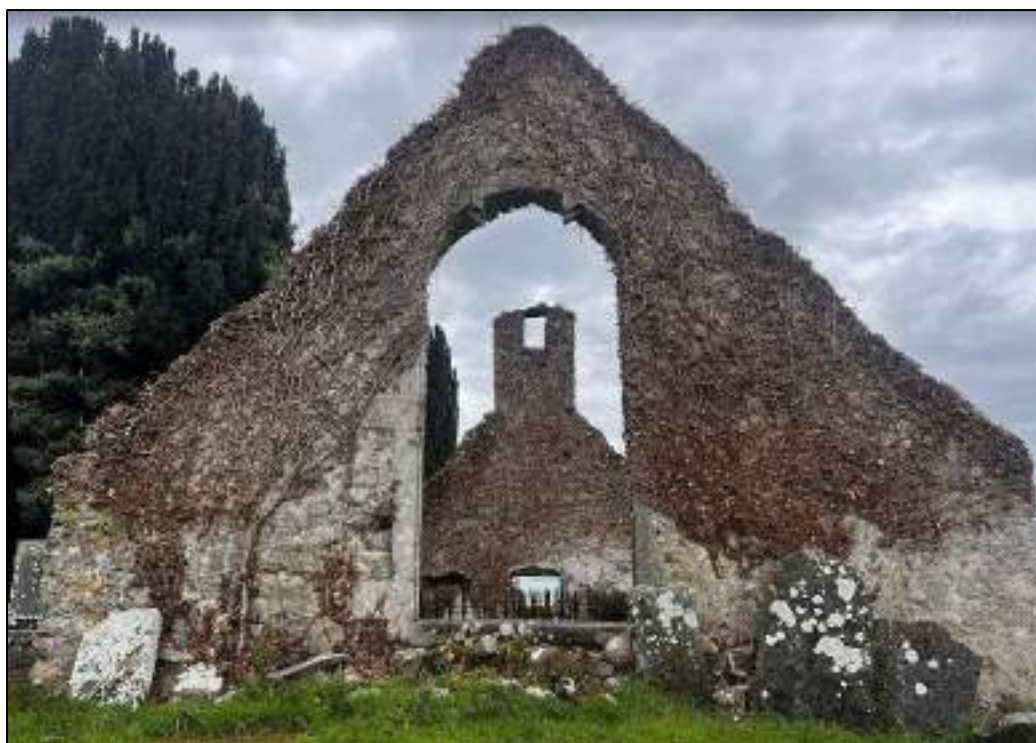
Plate 51: Donard Church after the removal of vegetation facing west with view of west gable, central door and bellcote..
