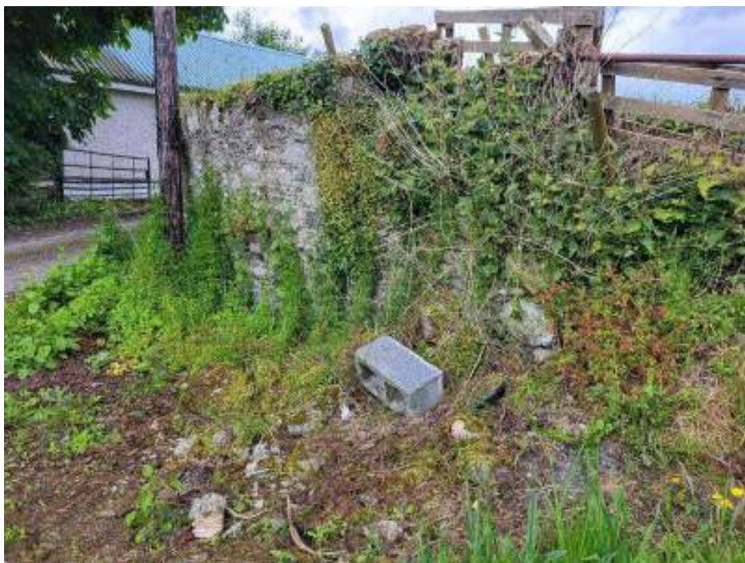
18. Graveyard wall leaning out at the south-west corner
