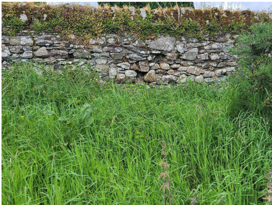
20. South Graveyard wall. (Note local damage)
