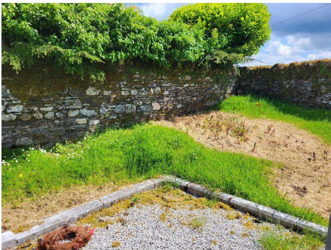
23. East Graveyard wall (Note severe leaning)
