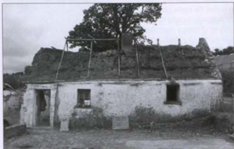
Fig 5 - Thatched roof exposed after the removal of the tin roof of a farmhouse at Castlekevin.
